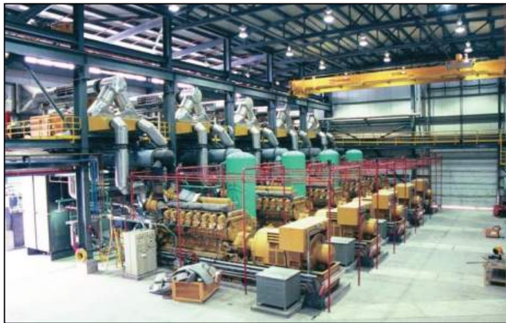
Heat recovery on Diavik diamond mine diesel powerplant #1
