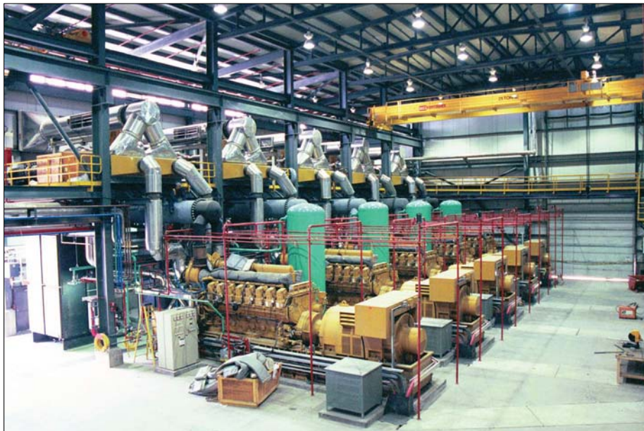
5 x 4.4MW power, Diavik diamond mine, NWT
