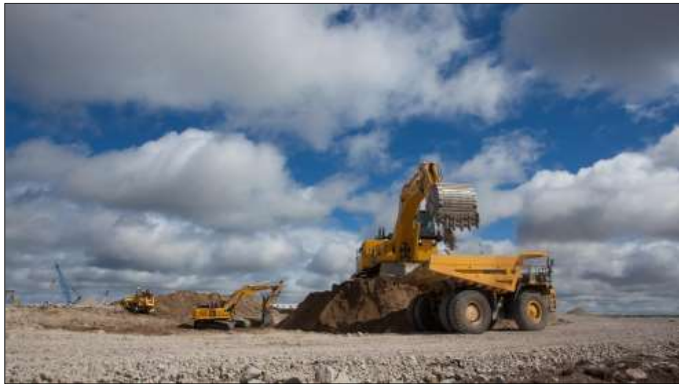
Heavy equipment in the Gahcho Kué quarry supports pre-development work at the site. Courtesy De Beers Canada.
