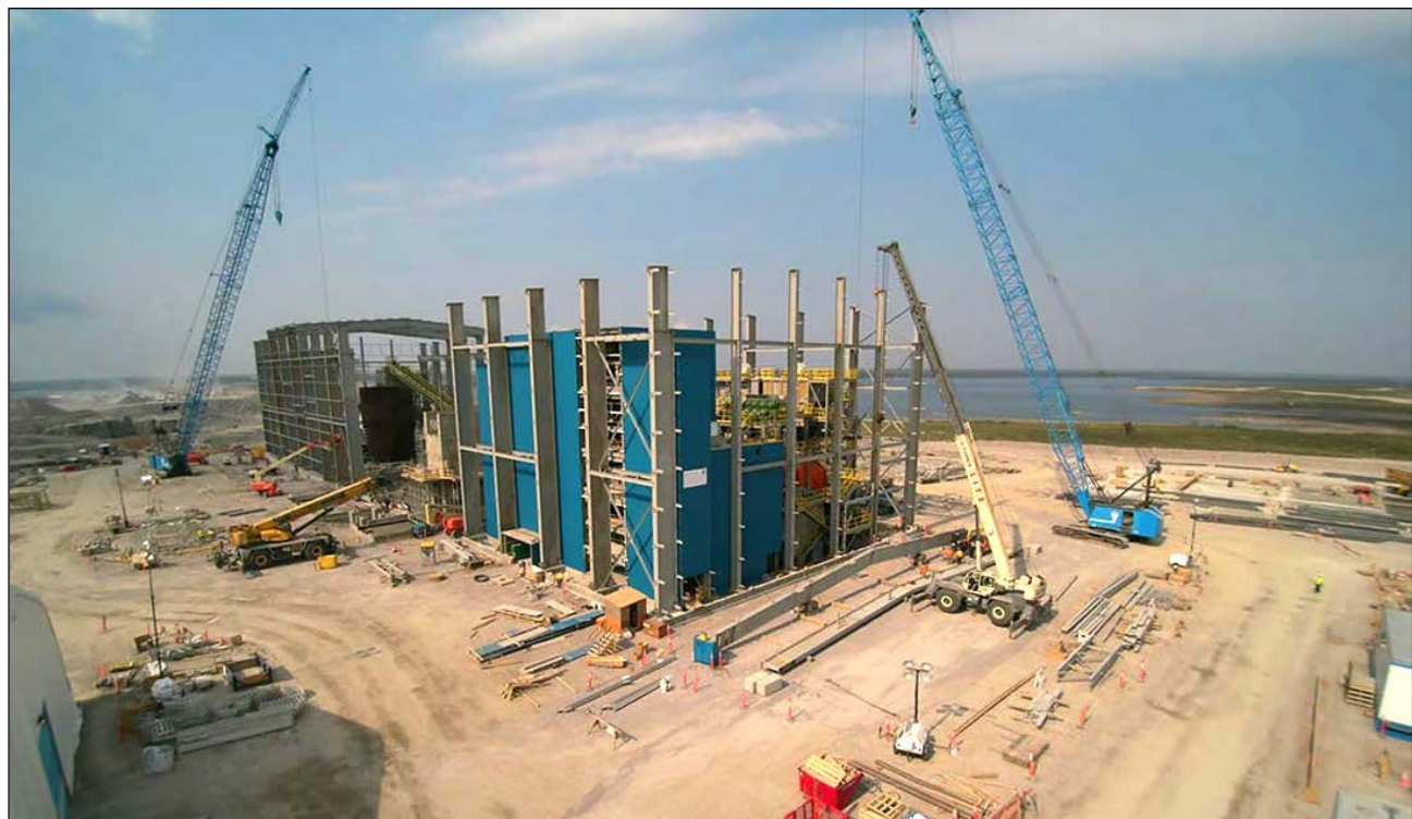
Construction of the NWT's newest diamond mine, Gahcho Kué, is now 70% complete. (Photo courtesy Mountain Province Diamonds)
