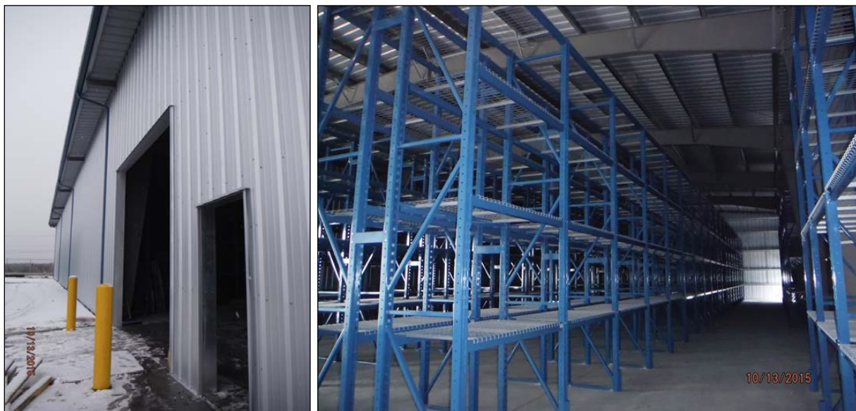
Work is progressing on the new NWT geological materials facility in Yellowknife.
