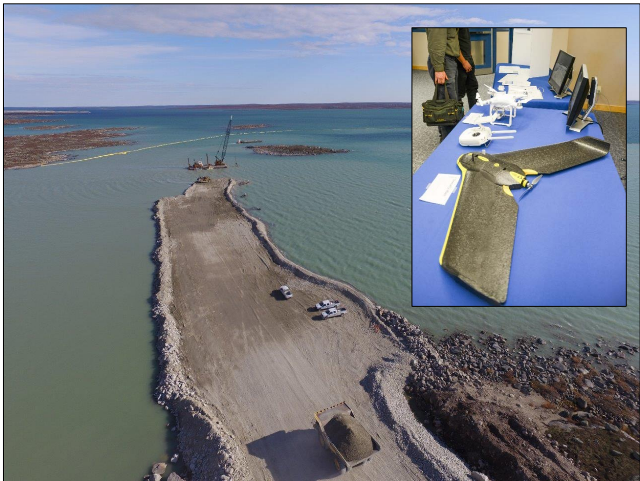
Aerial view of Diavik's A21 dike construction taken by drone (inset shows quadcopter and flying wing drones). Courtesy Diavik Diamond Mines Inc.
