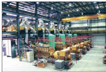
Heat recovery on Diavik diesels
