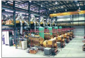
Heat recovery on Diavik diesels
