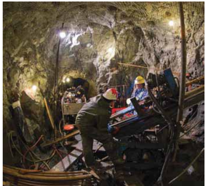
There is 4 km of underground workings from when the project was previously explored and mined. They allow year round drilling and access to massive sulphides. Photo courtesy of Prophecy Platinum.
